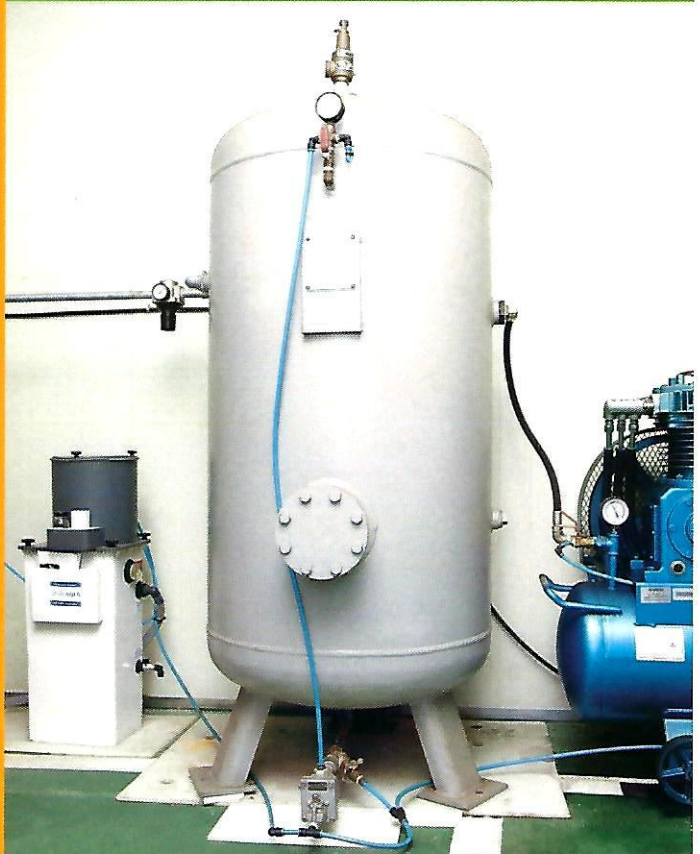
Receiver tank (Should install balance line)
